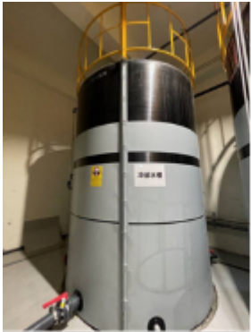
Cooling tower wastewater recovery
