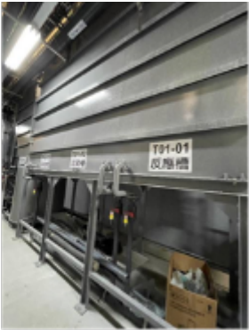
High hardness wastewater removal system
