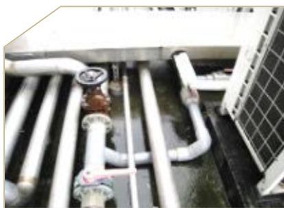
↑ Factory Rain water recycling system integration
