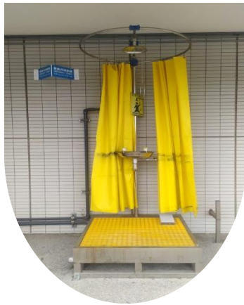
Emergency shower equipment in water treatment areas
