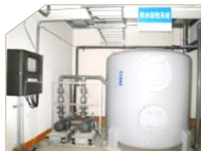
↑ Factories installed with rainwater recycling system
