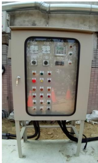
Discharge monitoring and control panel
